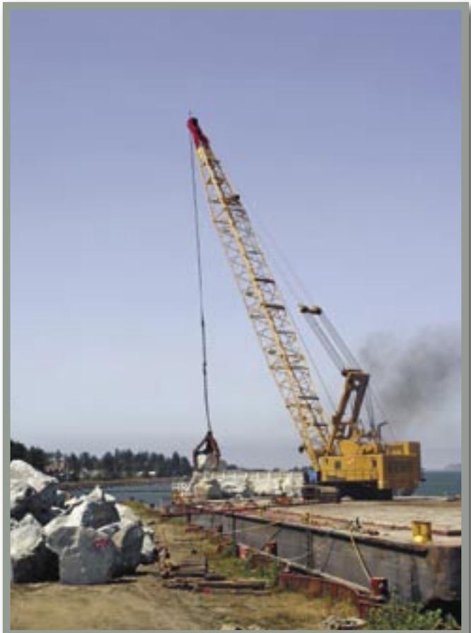
A second Manitowoc 4600 Vicon crane offloads rocks from the Kiewit barge at the Nygard Logging dock in Warrenton, Ore.
